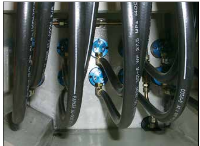
DEUBLIN 1117 Bearingless Unions on Automotive Transfer Line
