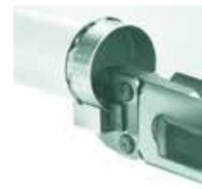
Repeat the operation until the required minimum of lugs for each diameter have been achieved.
