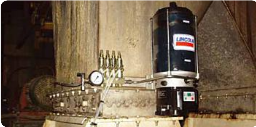
This Centro-Matic automatic electric pump and injectors are lubricating bearings in a very abrasive and dusty environment.
