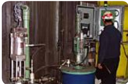
These Lincoln pumps deliver grease directly from a 400 lb. (181 kg) drum to 200 SL-V injectors located approximately 250 ft. (61 m) away in a steel mill.
