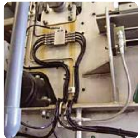
In this corrosive environment, a stainless steel Lincoln Quicklub system is lubricating and purging 32 points on a belt press in a wastewater plant.
