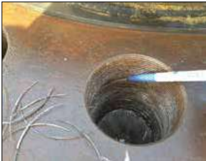
▲ A typical thread before refurbishment
