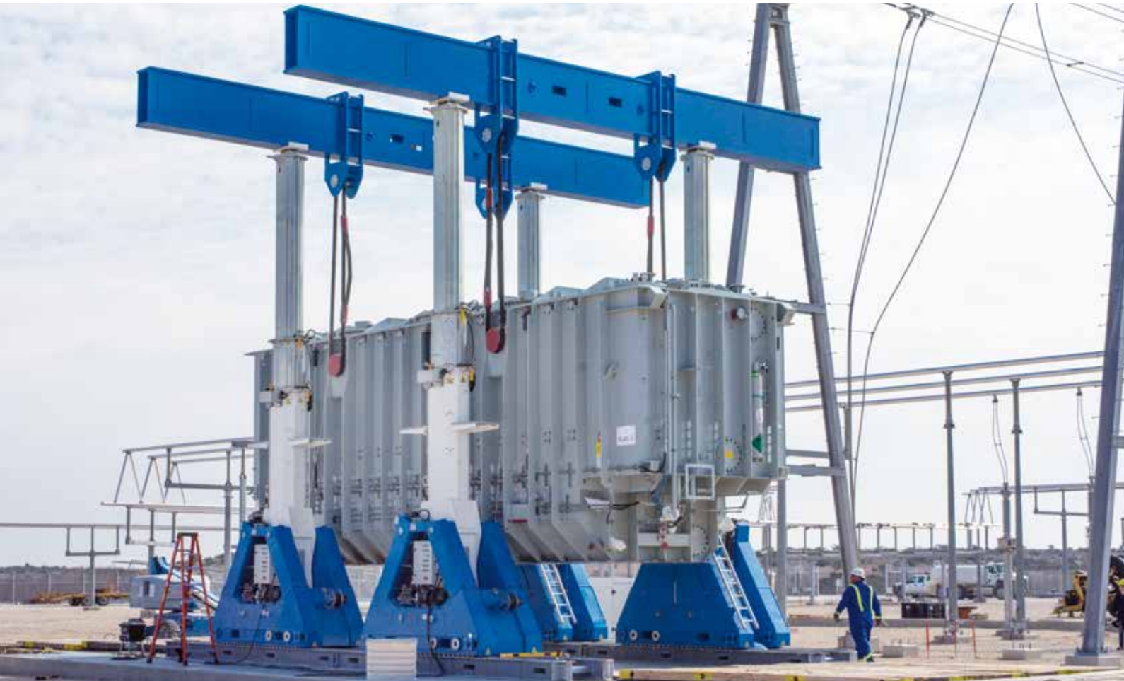
An SBL900 hydraulic gantry was used to transfer the transformer from the rail car to the heavy haul truck. Upon arriving at the sub-station, the hydraulic gantry was utilized to install the transformer on its platform.
